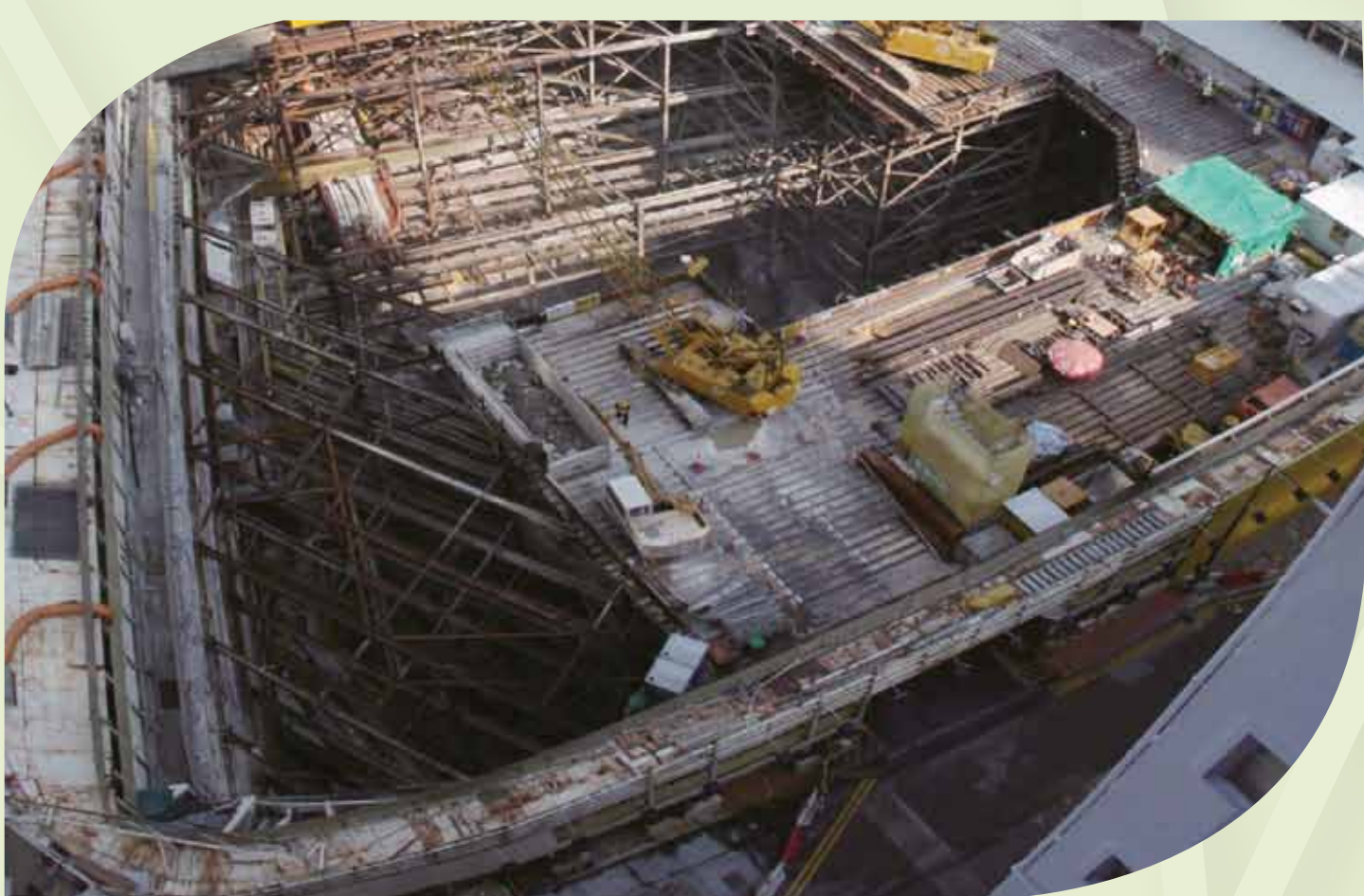
於圍街板上安裝通風機以改善工地週邊的空氣質素 Installation of ventilation fans along the hoarding to improve air quality outside the site
