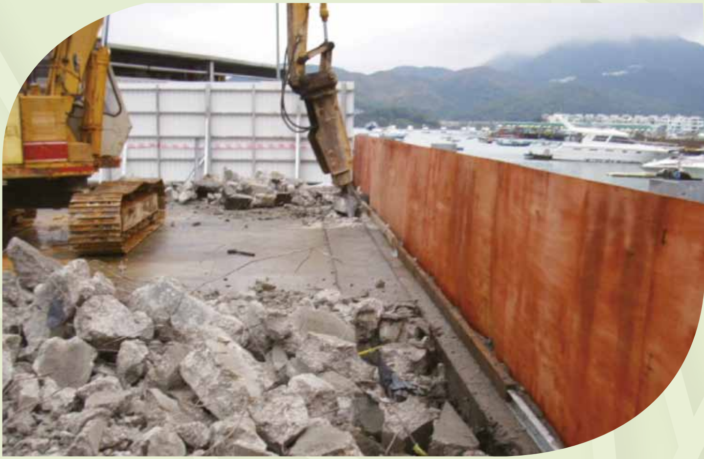
於工地範圍設置夾板及混凝土，防止污水流入大海。 Setting up plywood and concrete at the site boundary to prevent waste water from going into the sea.
