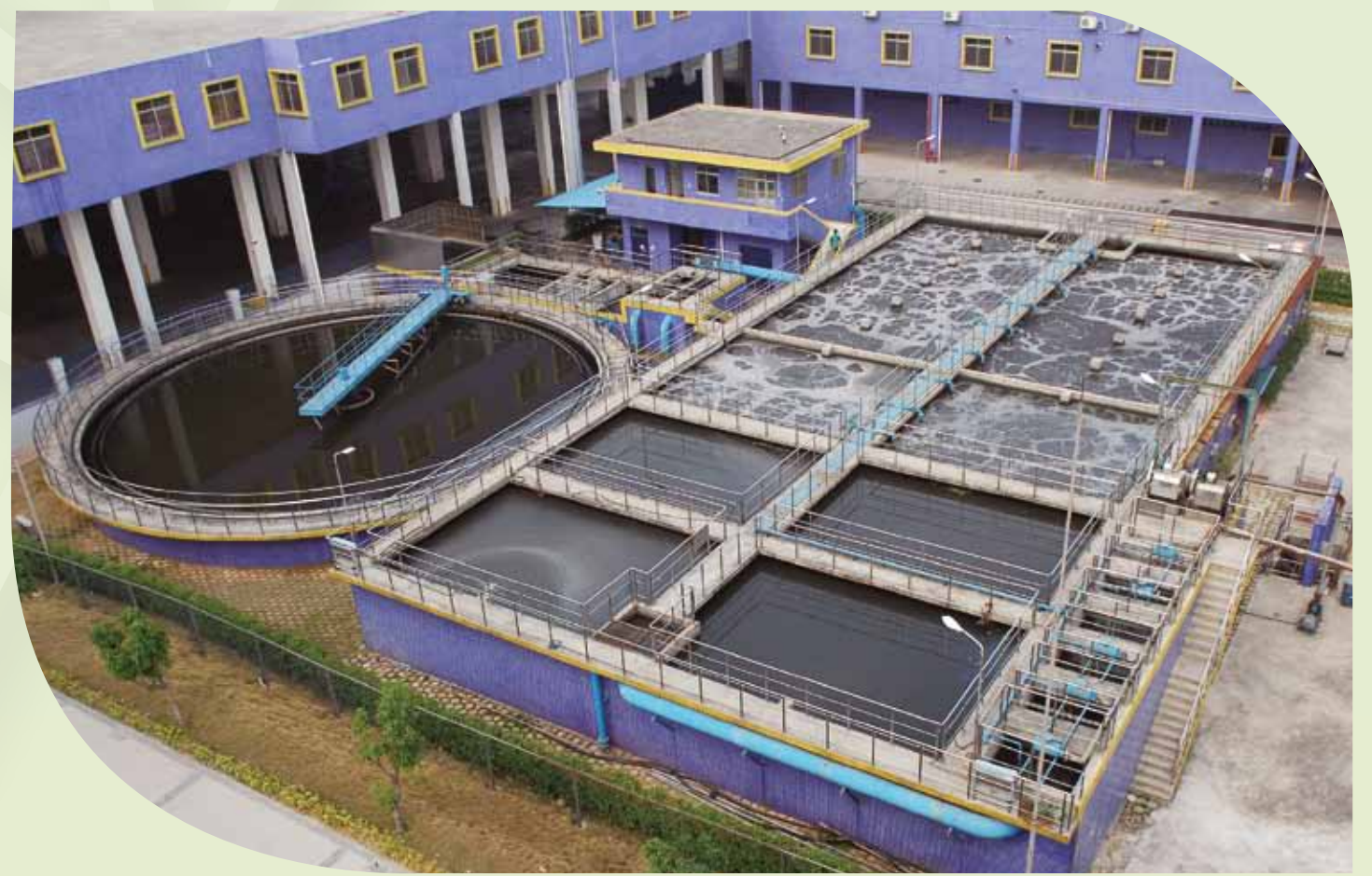
廠房設有三座污水處理廠 The 3 Wastewater Treatment Plants on site
