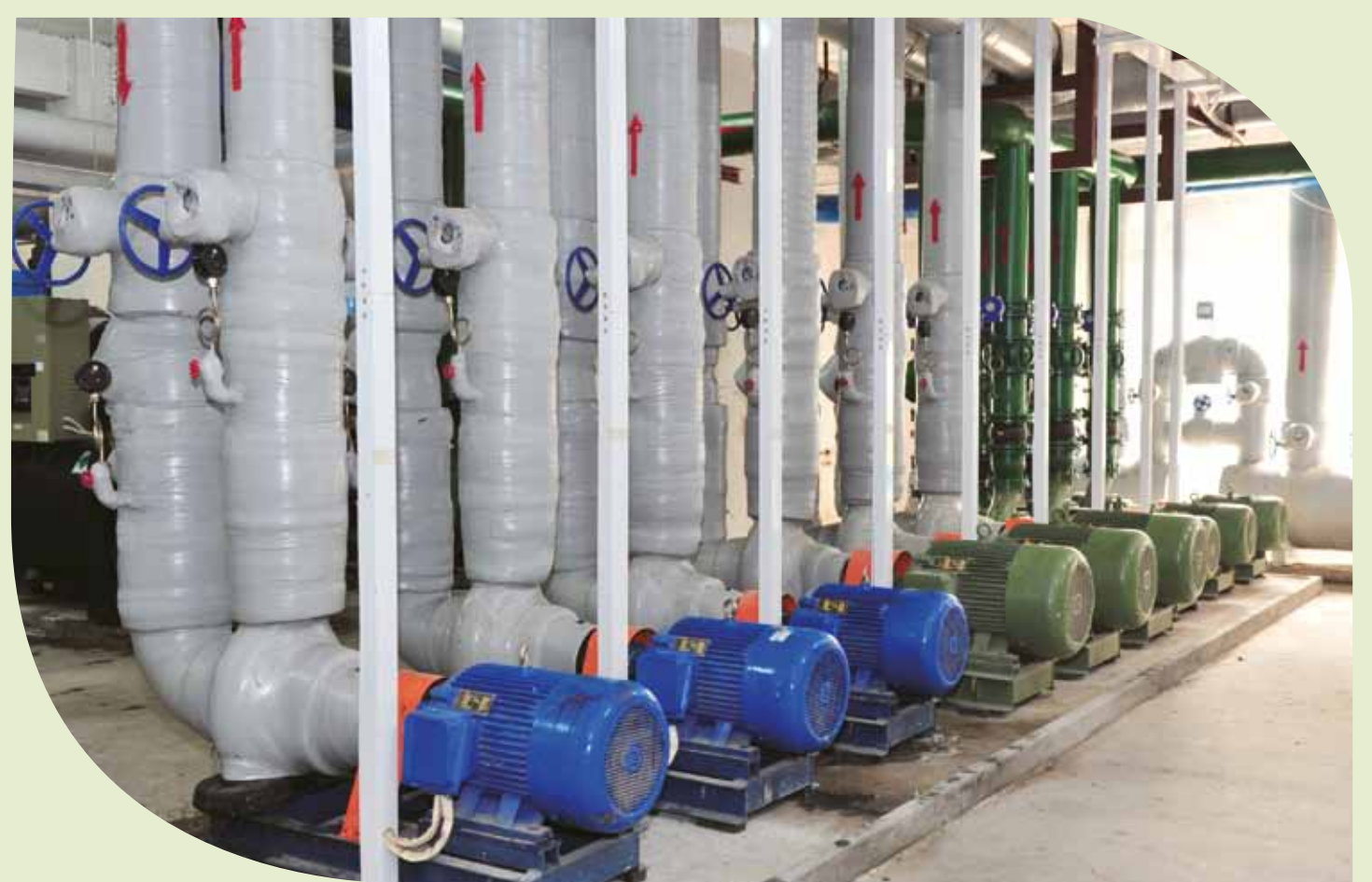
冰蓄冷系統 Slurry Ice Air-conditioning System
