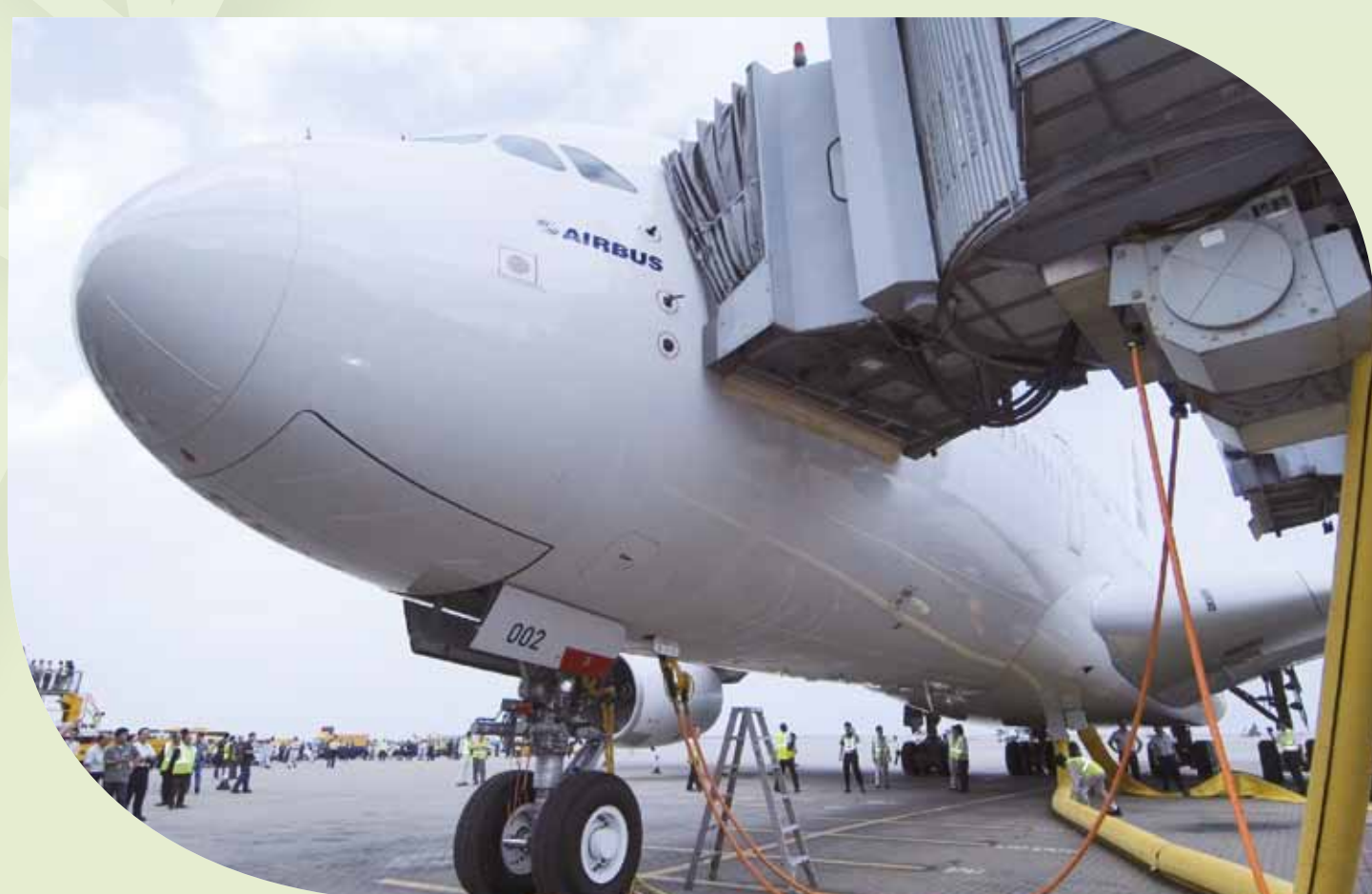
為客機提供固定地面供電系統及預調空氣系統 Provision of fixed ground power and pre-conditioned air systems to aircraft
