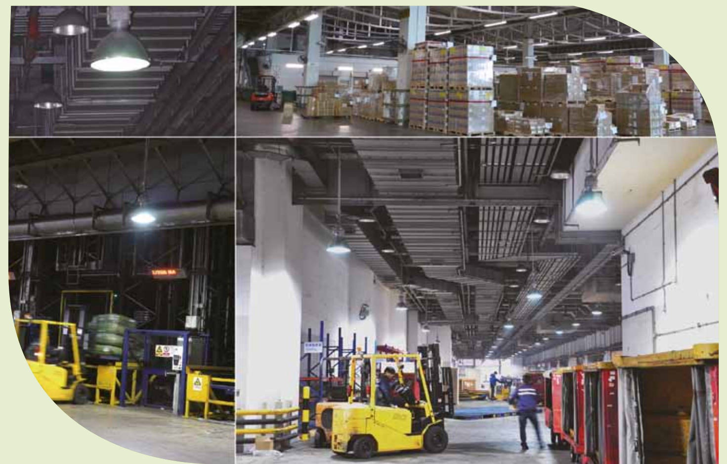
我們把逾六百套鹵素燈更換成電磁感應照明燈及節能日光燈，以節省能源消耗多達百分之五十。 Over 600 sets of Hi-Bay lights were replaced by energy-efficient induction lamps and fluorescent lights with more than 50% of energy saved.
