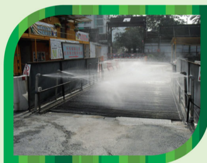
自動洗車池使用循環水 Automatic wheel-washing facilities using recycled water
