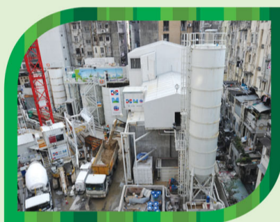
挖掘出來的物料及泥漿經由泥漿處理廠處理。處理後的泥漿/水會循環使用。 Excavated material and slurry are treated by the Slurry Treatment Plant. The treated slurry/water will be recycled.
