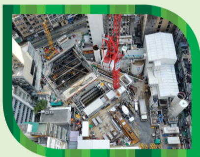
西湖里工地已興建可減少50分貝的隔音罩 Noise enclosure at Sai Woo Lane which reduced noise by 50dB
