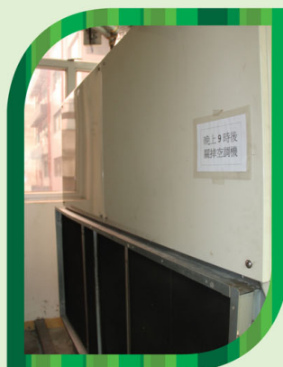
非繁忙時間冷氣控制及定期維修保養 Non-peak hour control & regular maintenance of air-conditioning
