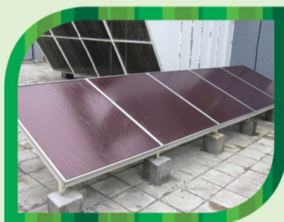
已加裝太陽能發電系統，以提供大廈部份電力。 Our electricity supply is partially provided by solar energy system.
