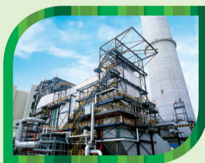
港燈是除日本外東南亞地區首間為旗下發電機組安裝煙氣脫硫裝置的電力公司。 HK Electric was the first power company in South East Asia, except Japan, to install a Flue Gas Desulphurization system in its generating units.
