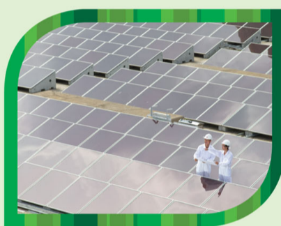
由5,500塊薄膜太陽能光伏板所組成的550千瓦容量太陽能發電系統，是全港同類型中規模最大的裝置。 The 550 kW solar power system, comprising 5,500 Thin Film Photovoltaic (TFPV) panels, is the largest of its kind in Hong Kong.
