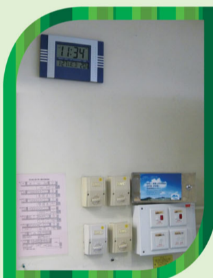
課室內裝設電子溫度計，以符合空調溫度設定在攝氏25.5度 Thermometers are installed in classrooms in order to keep the room temperature at around 25.5°C
