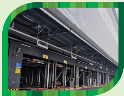
把頂篷區的二百瓦特傳統日光燈更換為五十八瓦特的T8日光燈，節省的電量高達百分之七十一。 200W canopy lamps in the canopy area were replaced by 58W T8 fluorescent tubes saving 71% of energy.
