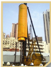
在進行撞擊式打樁時，特別加裝雙層隔音屏障，總噪音量約減少了15分貝。 Additional acoustic barrier was incorporated with Acoustic Enclosure in percussive piling. Total noise reduction was about 15 dB(A).
