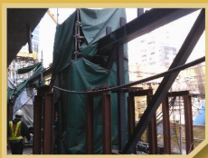
施工期間使用隔音墊，以減少噪音對附近居民的影響。 During construction, acoustic mats were used to minimize noise impacts to nearby residents.
