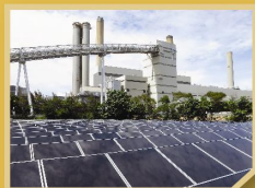
南丫發電廠大塘新發電系統於二零一三年三月擴增至一兆瓦，是香港目前最大規模的太陽能發電系統。 The Solar Power System in Lantau Power Station was extended to 1MW in March 2013, and is by far the largest solar system in Hong Kong.
