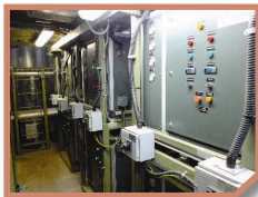
熱泵系統利用空調系統之廢熱能將水加熱，供應全院熱水，例如廚房及浴室。每年可減少排放於大氣層之空氣污染物質如二氧化碳、二氧化硫及氮氧化物約2000噸。 Heat pump system recovers waste heat energy from the air-conditioning system and supplies hot water to the hospital, including kitchens and bathrooms. This helps reduce 2000 tonnes of air pollutants such as carbon dioxide, sulfur dioxide and nitrogen oxides emitted to the atmosphere.
