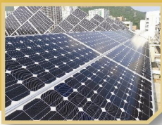
天台上的太陽面板，能自動追蹤光源。 Roof-mounted solar panels which are sun tracking.
