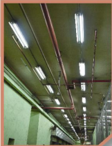
倉庫及寫字樓陸續將T8光管更換為T5光管。 T8 light tubes were replaced by T5 light tubes in the warehouse and office in phases.
